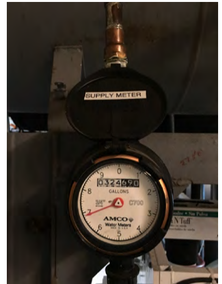
Cooling tower make-up meter.
